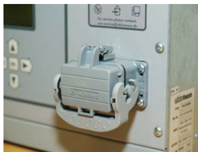
High voltage power outlet
